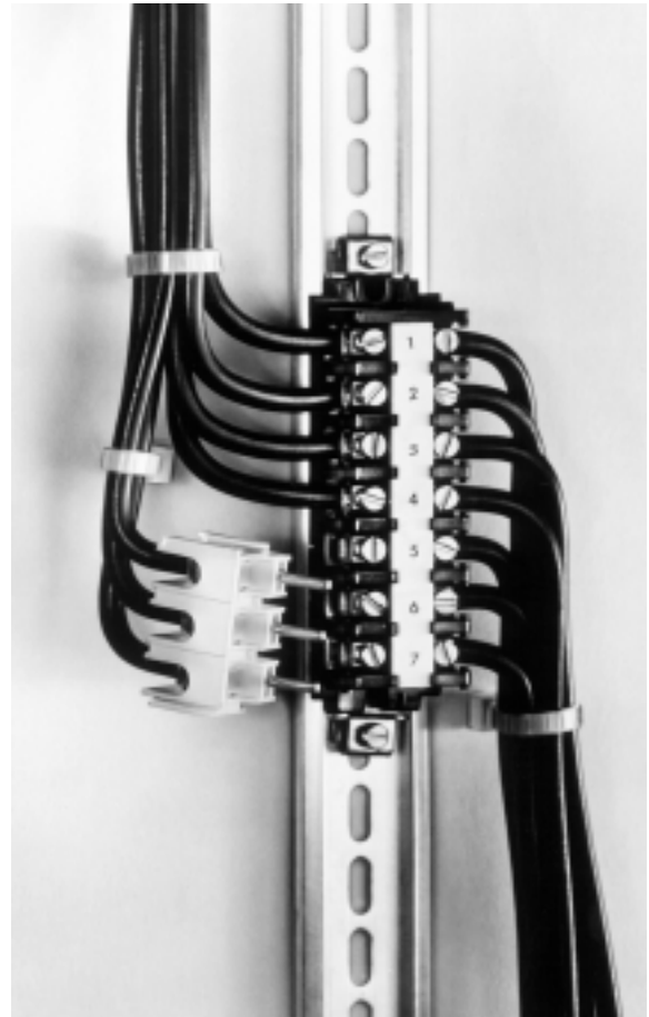
Group Circuits with Interlocking Fanning Strips
